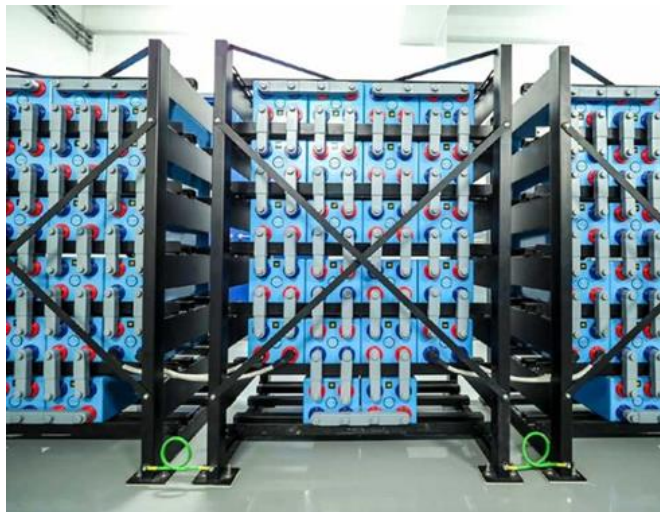
Fig. 4. Wellington battery energy storage system (BESS)
