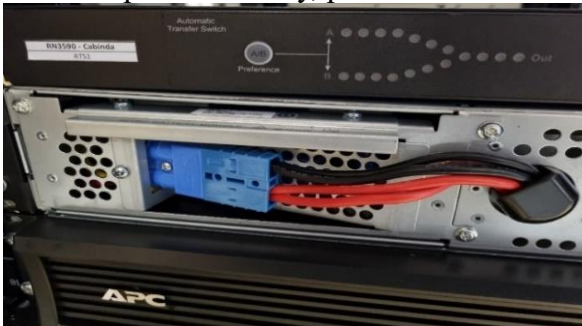
Fig. 1 – UPS battery connected
